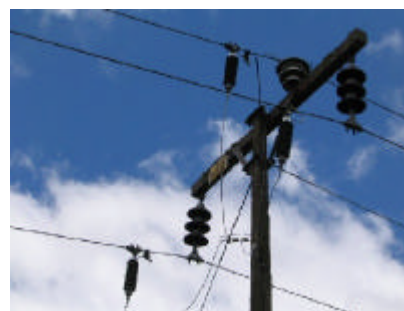
Fig 6.2 – 36 kV Brazilian ZnO Lightning Arrester
