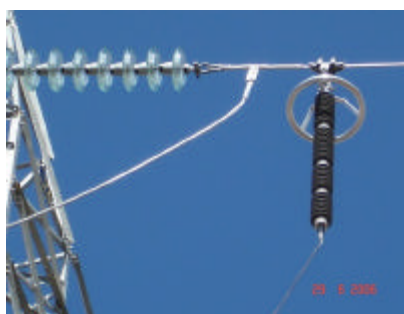
Fig 6.3 – 120 kV Brazilian ZnO Lightning Arrester
