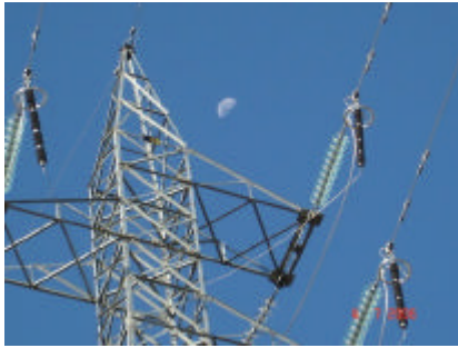
Fig 6.4 – 120 kV Brazilian ZnO Lightning Arrester
